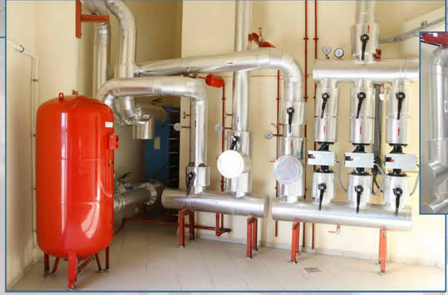
AT FIRST 34 Floors, One Block, 241 Flats, 32 pcs 125 kw wallhung boiler were used
